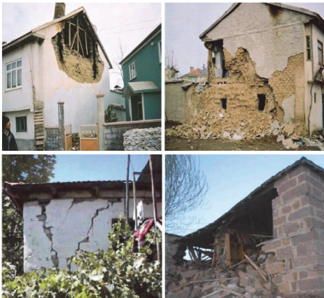
Figure.1 Damage to masonry structures
