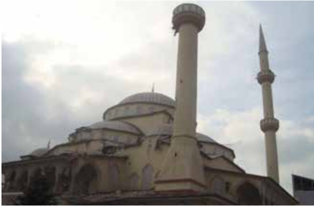
Figure 24. Intact and damaged minarets of a mosque in Van
