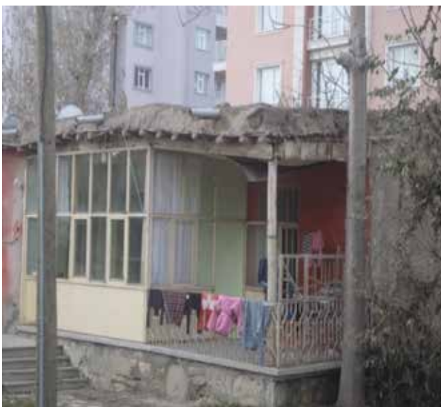
Figure 21. Excessive earthfill on the roof of a masonry building.
