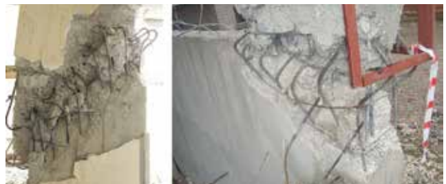
Figure 30. Shear damage and buckling of longitudinal reinforcement due to insufficient lateral rebar interval
