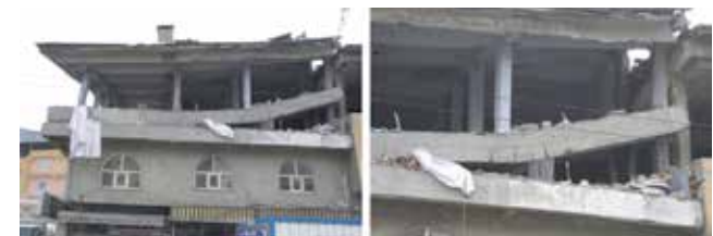
Figure 14. Partial collapse of the slab due to pounding in Erciş
