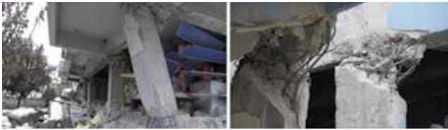
Figure 9. Examples of plastic rotations at the end of columns instead of beams in Erciş
