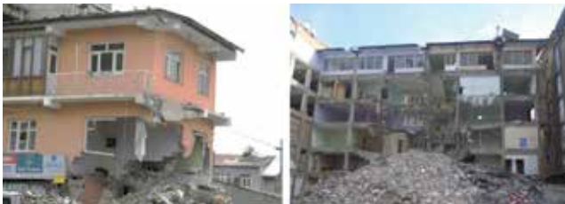
Figure 15. Damage due to the impact of the collapsed building on the neighbouring building in Erciř and Van
