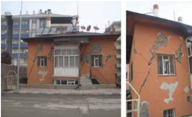
Figure 20. Typical shear damage observed on structural walls of a masonry building in Van
