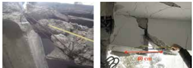
Figure 28. Inadequate lateral reinforcement intervals
