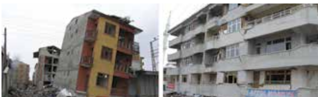
Figure 12. Collapse of two buildings due to soft storey effect at the ground floor level in Erciş
