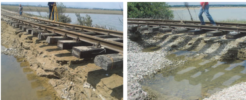
Figure 3. The state of the railway superstructure after the flood on the R105 Vinkovci – Drenovci – state border railway sections [17]
