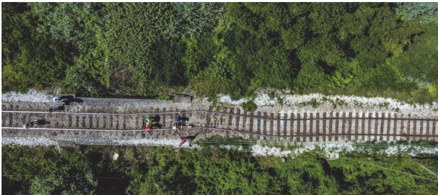
Figure 2. The condition of the M103 Dugo Selo - Novska railway section following the effects of high temperatures [18]
