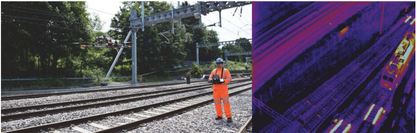
Figure 25. The use of drones and thermography to control the correctness of heaters on turnouts [114]
