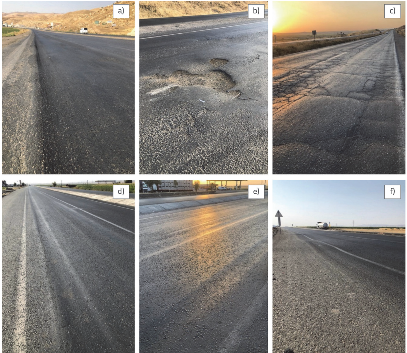
Figure 9. Damages in the old asphalt pavement: a) rutting and undulation; b) rutting, fatigue cracks and potholes; c) rutting, fatigue and block cracks, alligator cracks, damages in the new asphalt pavement; d, e, f) rutting damage and corrugation
