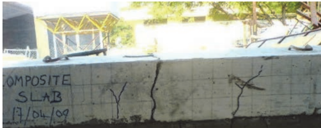
Figure 9. Composite panel after failure
