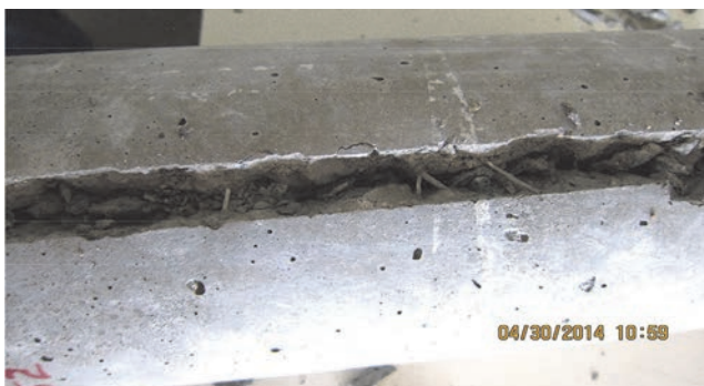
Figure 6. Fibres in concrete across crack section
